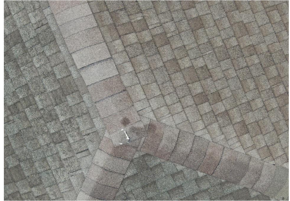
35. OPEN VOID IN RIDGE SHINGLE
