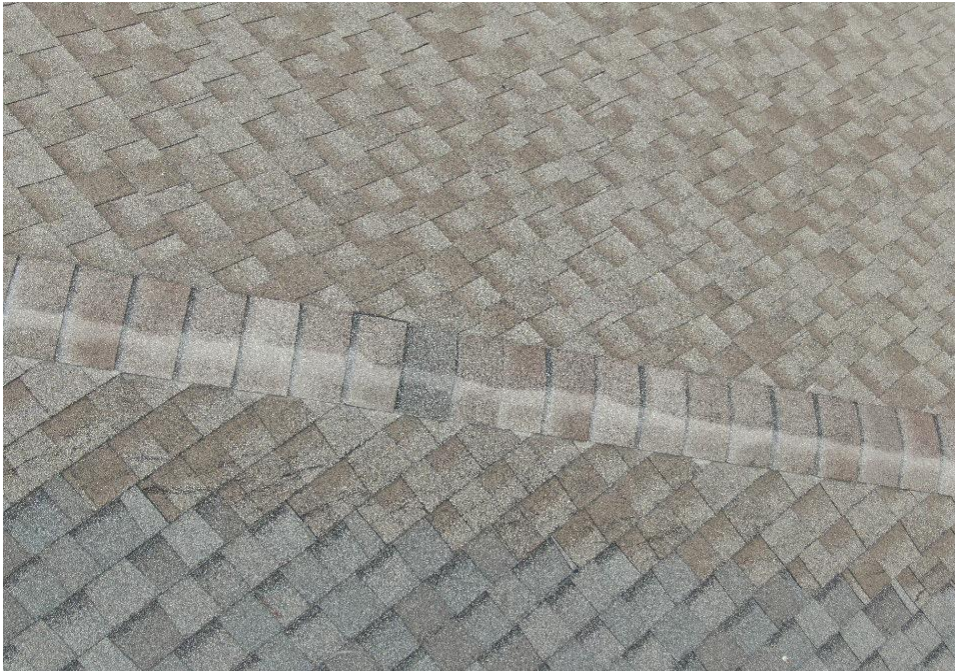
13. OVERVIEW OF CRACKED RIDGE SHINGLE
