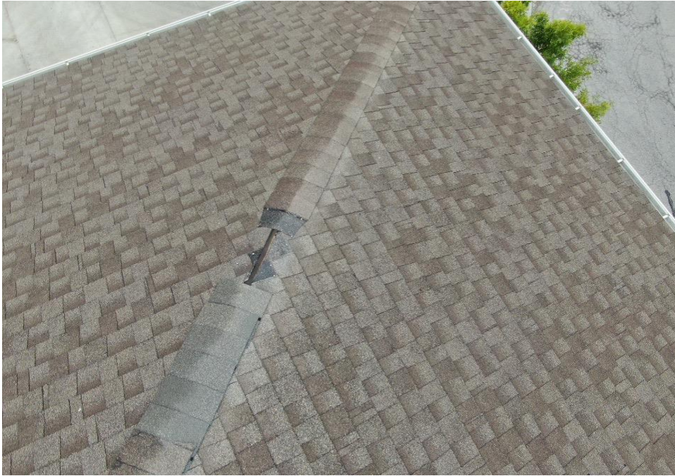
18. MISSING RIDGE SHINGLES
