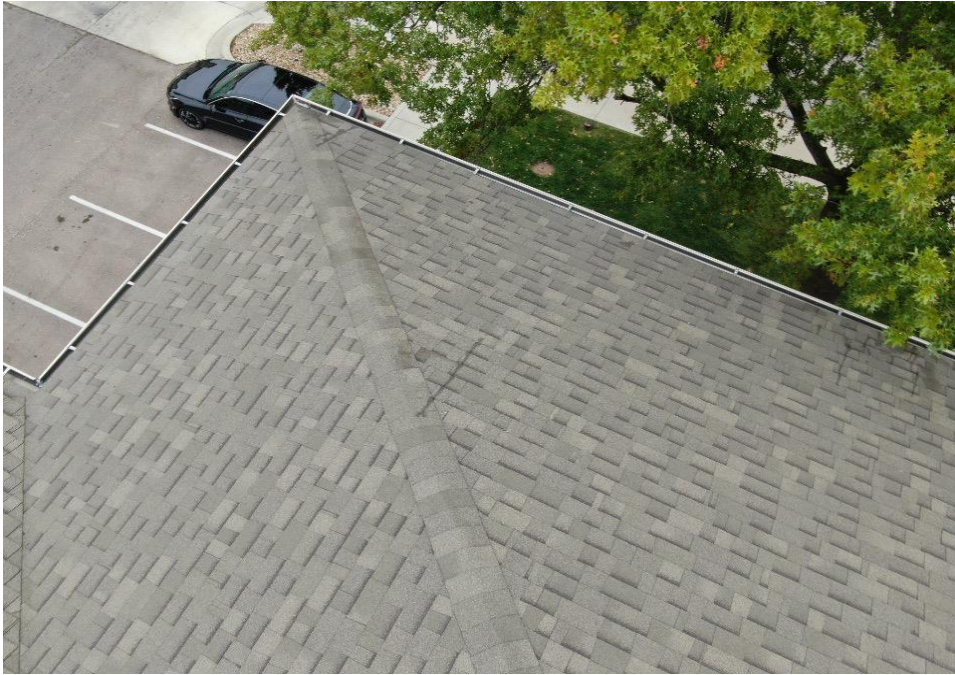
31. TREE LIMBS OVERHANGING ROOF/DEBRIS IN GUTTER
