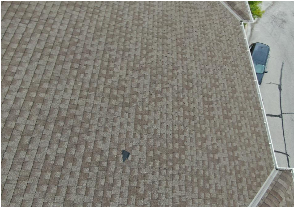
20. SHINGLE DEBRIS ON ROOF SURFACE
