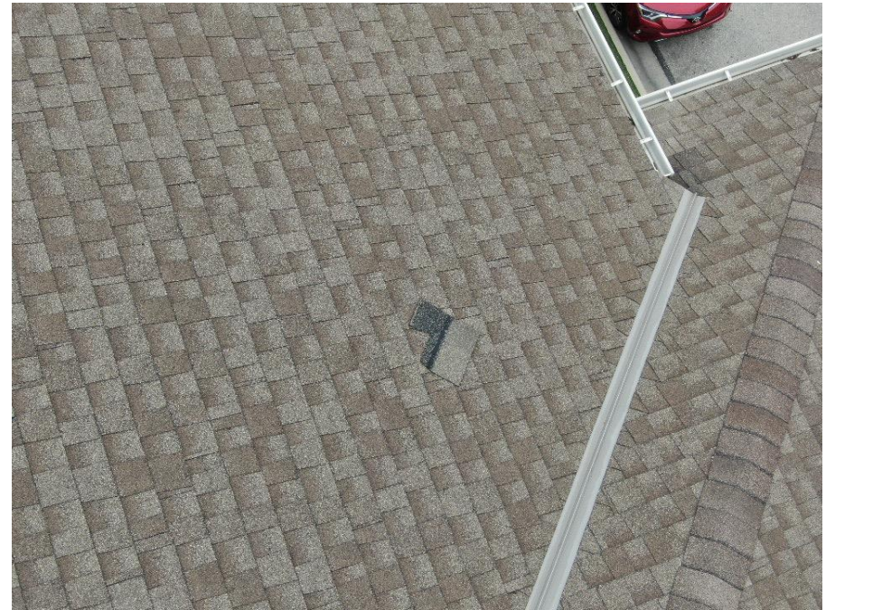
21. SHINGLE DEBRIS ON ROOF SURFACE
