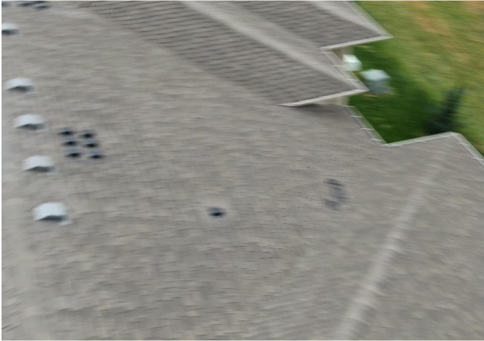
40. SHINGLE DEBRIS ON ROOF SURFACE
