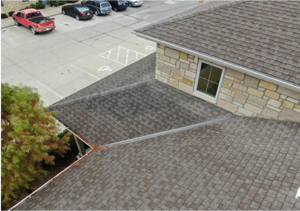
34. DEBRIS IN EXTERIOR GUTTERING
